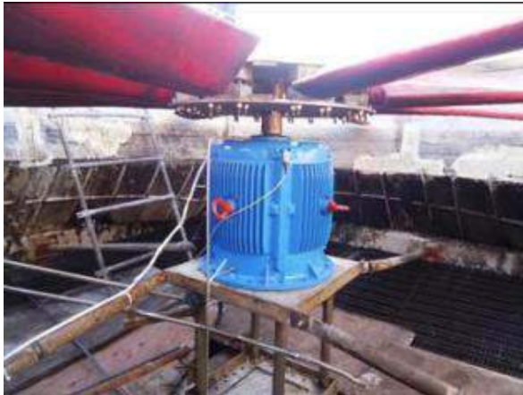
Figure 10. Cooling tower with PM motor
