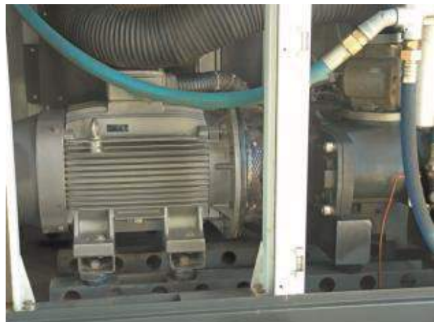
Figure 6. Compressor with PM motor
