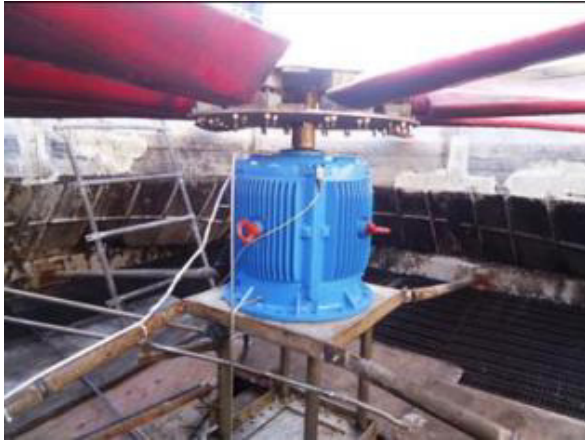
Figure 10. Cooling tower with PM motor
