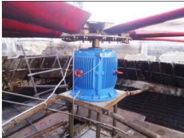
Figure 10. Cooling tower with PM motor
